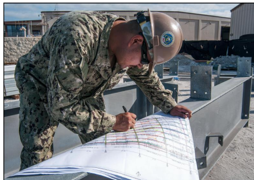
A servicemember looks over plans during the construction of a storage facility on Joint Base Pearl Harbor-Hickam, Hawaii.
