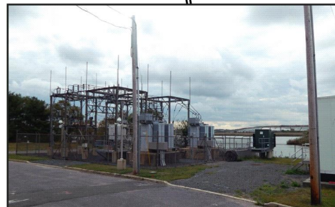
Pumping station power grid
