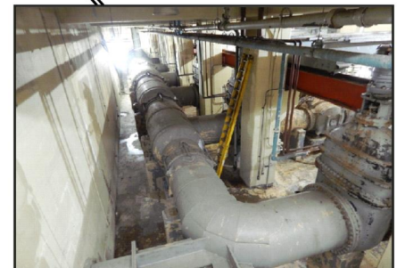
Main pumps and discharge pipe
