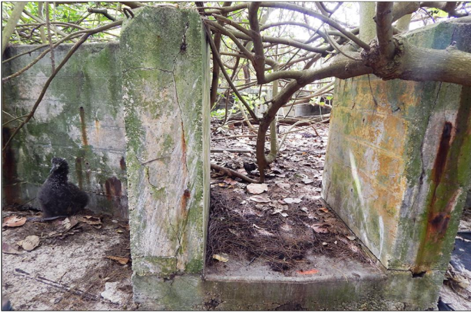
Figure 39: Battery A, 5-Inch Gun Position (Property No. S-9), Midway Atoll, Sand Island (April 15, 2015)
