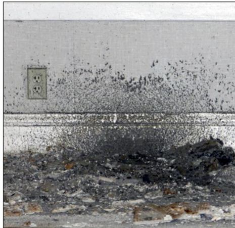
Portions of the ceiling have collapsed, spraying debris on to the floors and walls.
