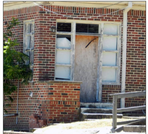
Exterior view of the building shows broken windows and missing bricks.
