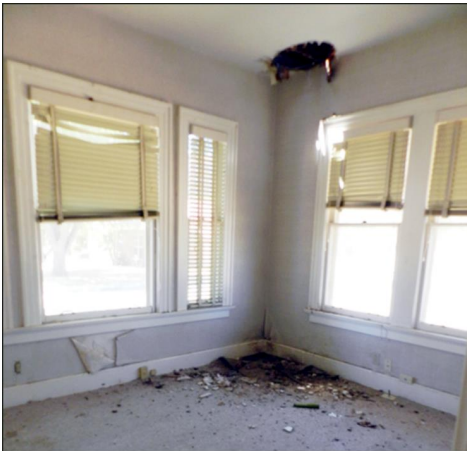
Interior damage of Kerrville Medical Center.
