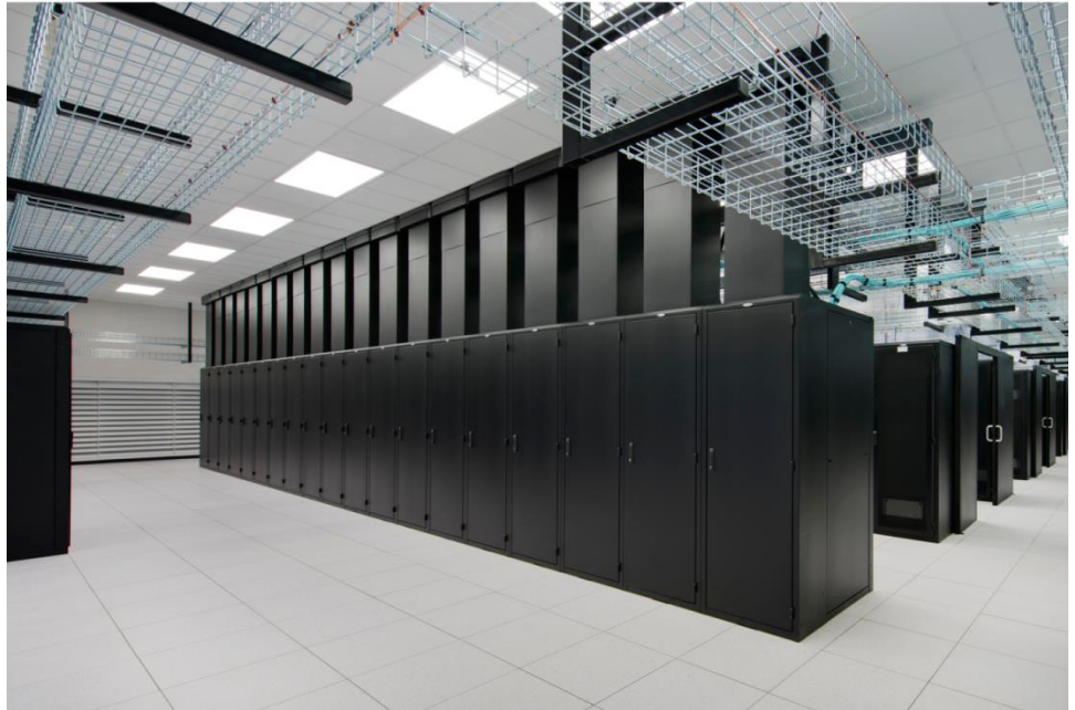
Figure 1: Example of Data Center Server Racks at the Social Security Administration's National Support Center
