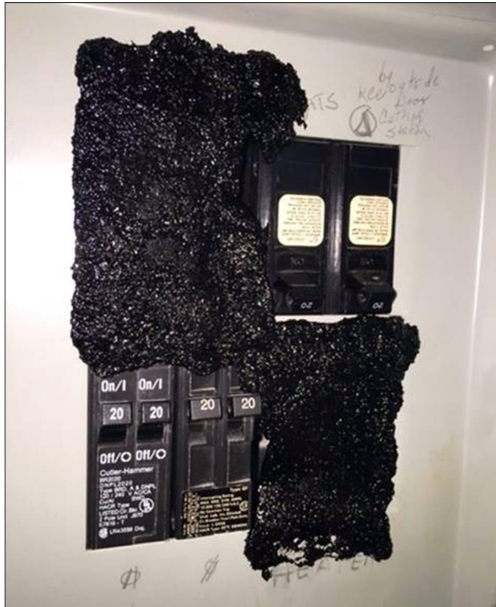
Figure 3: Non-Industry-Standard Repair to an Electrical Panel Identified During a Real Estate Assessment Center Physical Inspection
