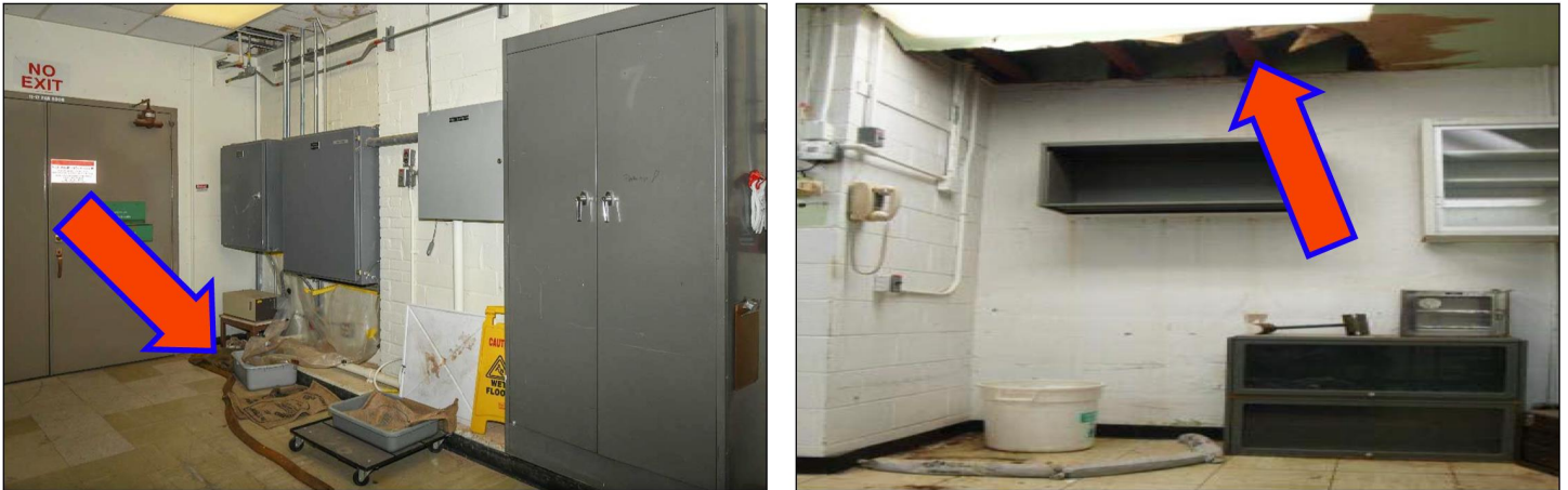
Figure 4: Weather Damage in the Analytics and Chemistry Laboratory at the Pantex Plant
