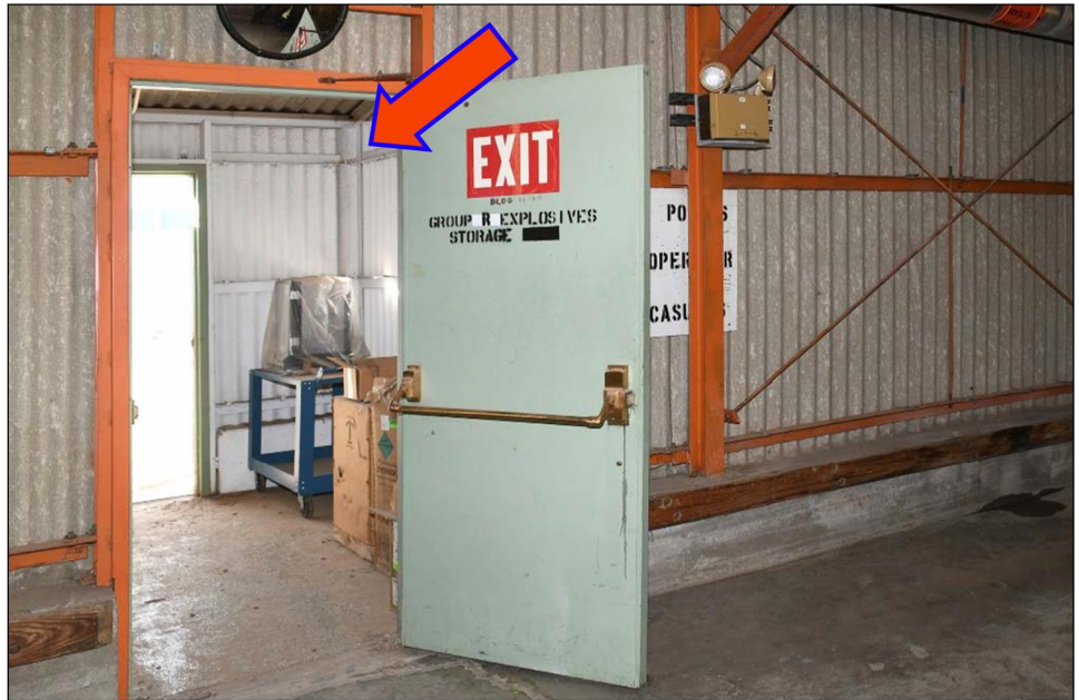
Figure 6: Inert (Non-explosives) Storage Closet at Pantex Plant that Is Characterized as an Explosives-Related Asset
