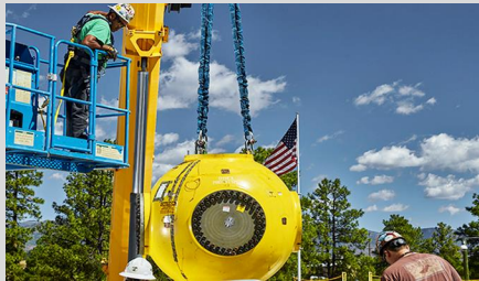
Steel vessel at Los Alamos's DARHT facility.
