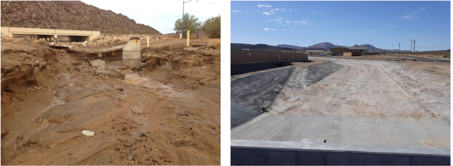
Figure 3: Flood Damage and Stormwater Diversion Channel at Fort Irwin, California
