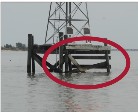
This damaged range/tower has been deemed unsafe to climb by an aids to navigation team.
