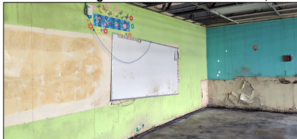
Classroom with molded floors and water damage on the walls at a school in San Juan, Puerto Rico.
