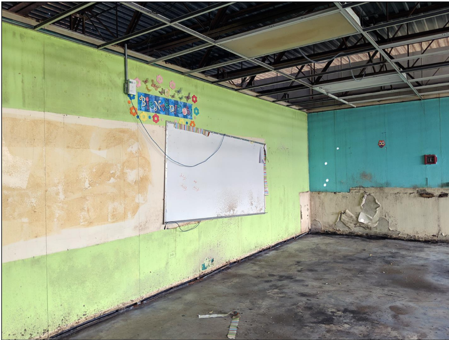
Classroom with mold on floors and water damage on the walls at a school in San Juan, Puerto Rico.
