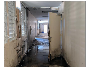
Interior damages to a school in Puerto Rico from water infiltration with standing water and molded walls.
