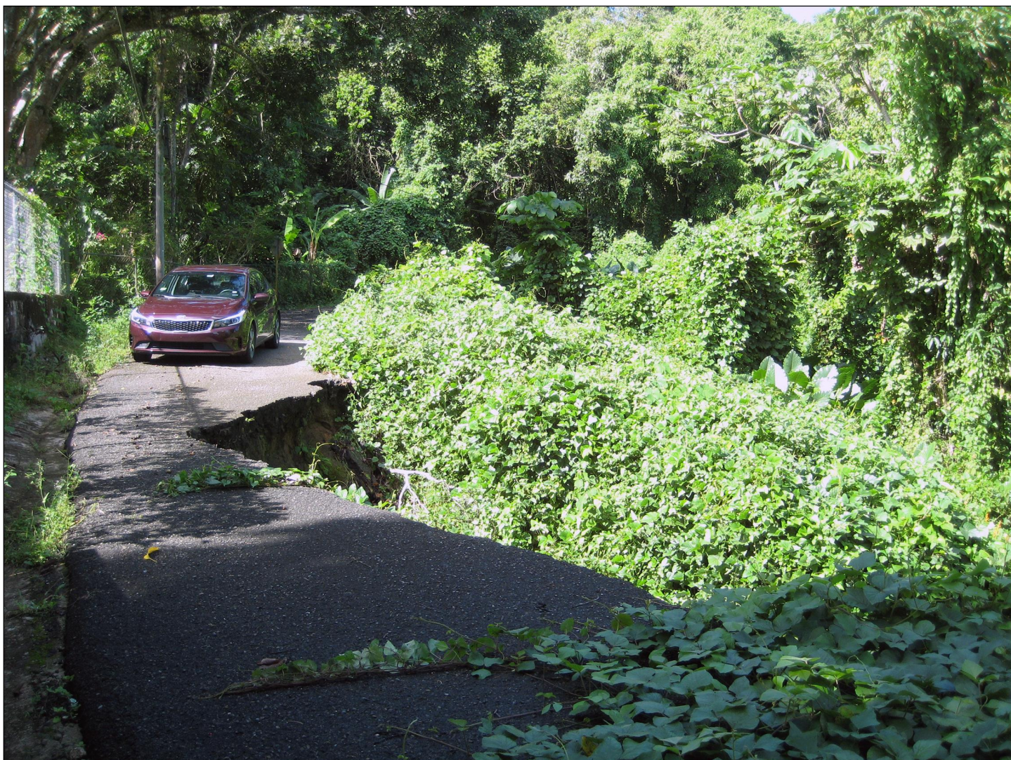
Figure 8: Collapsed Segment of Road near Maricao, Puerto Rico, September 2018
