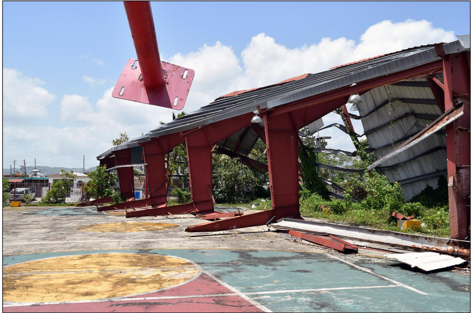
Figure 6: Damaged Sports Complex in Caguas, Puerto Rico
