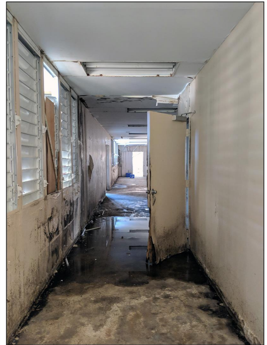
Interior damages to a school in Puerto Rico from water infiltration with standing water and mold on walls.
