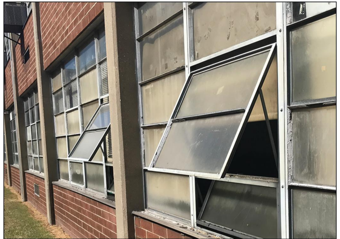
Open windows at a Maryland school without air conditioning in most areas of the building. The school district must close school if the building temperature rises above a safe level for students and staff.
