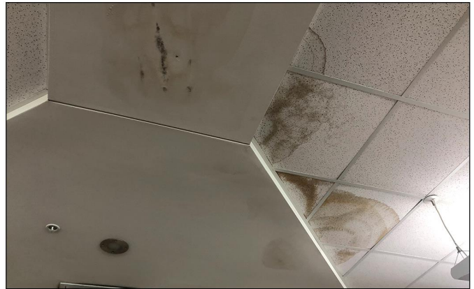
Water damage from HVAC leak in a Michigan school library
