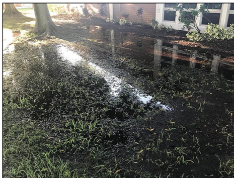
Standing water after a storm outside a school in Florida. School personnel work to clear drains and place sandbags in an attempt to mitigate water intrusion and flooding.
