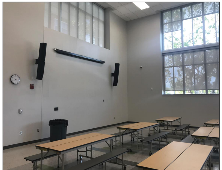
A projector and speakers for showing movies and playing music in a renovated cafeteria in a school in Maryland.
