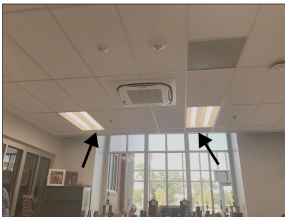
Light emitting diode (LED) lighting in a Maryland school
