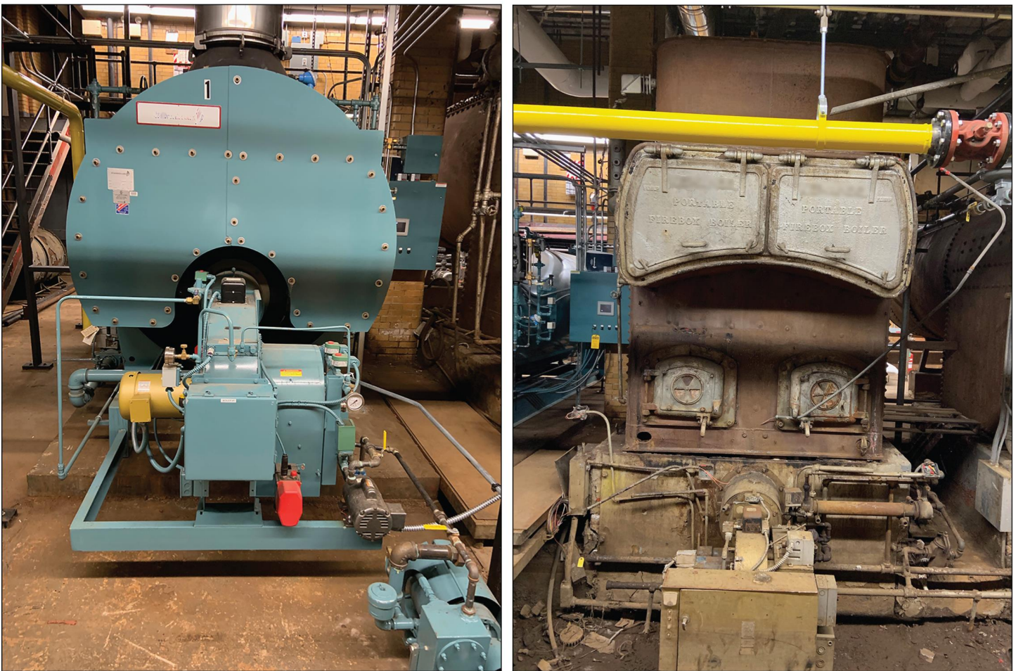
Figure 3: Public School in Rhode Island with One New Boiler (left) and One Original to 1931 Building
