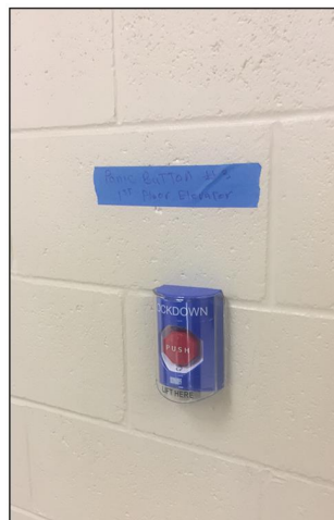
A button that locks exterior doors in the hallway of a Florida school.
