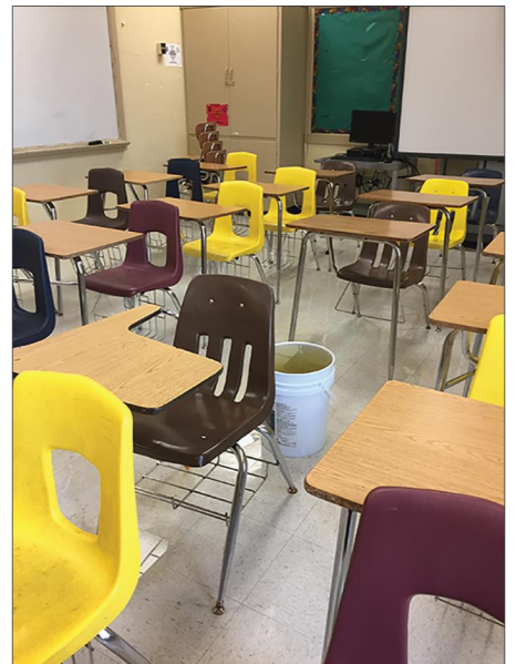
Bucket full of water in the middle of a Florida classroom with a roof leak.
