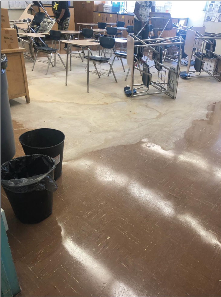
Water damage from HVAC leak in a California school, whose officials said replacing flooring is difficult because of asbestos floor tiles.
