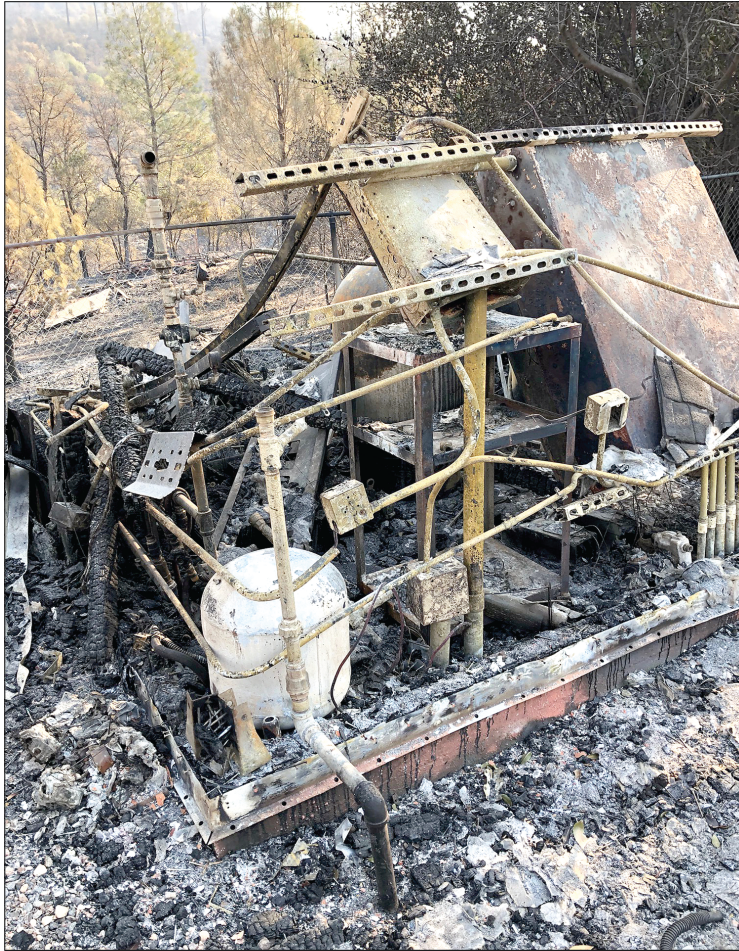
Figure 2. School Water System Damaged by the Camp Fire in 2018
