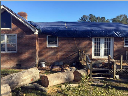
Roof and Interior Damage to a Survivor’s Home as a Result of Hurricane Florence
