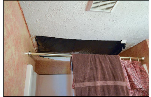
A survivor patches a leak in her home with a trash bag nine months after Hurricane Michael caused a tree to fall on her house.
