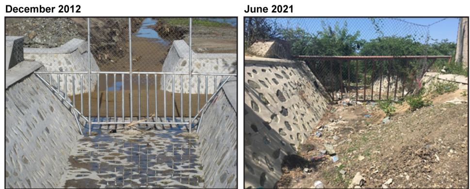
Figure 12: Comparison of USAID-Funded Drainage Channels at Caracol EKAM Housing Development Site in Haiti in December 2012 (left) and in June 2021 (right), Showing Buildup of Debris
