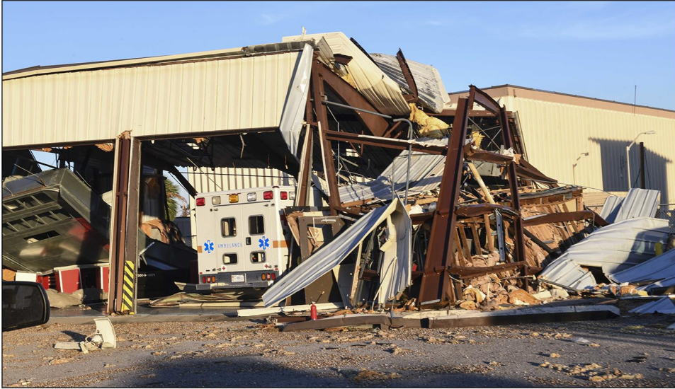
Figure 7: Hurricane Michael Damage at Tyndall Air Force Base in 2018
