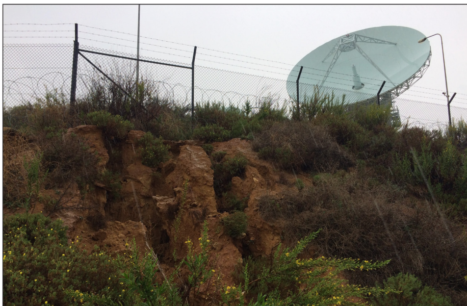
Figure 7: Hillside Impacted by Erosion at a Department of Defense Installation in Europe
