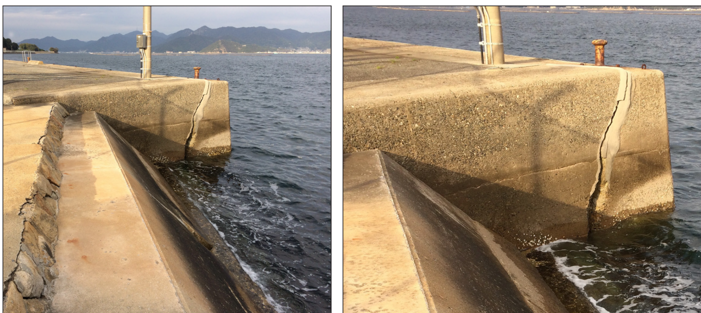
Figure 10: Damaged Seawall at a Department of Defense Ammunition Depot in the Pacific
