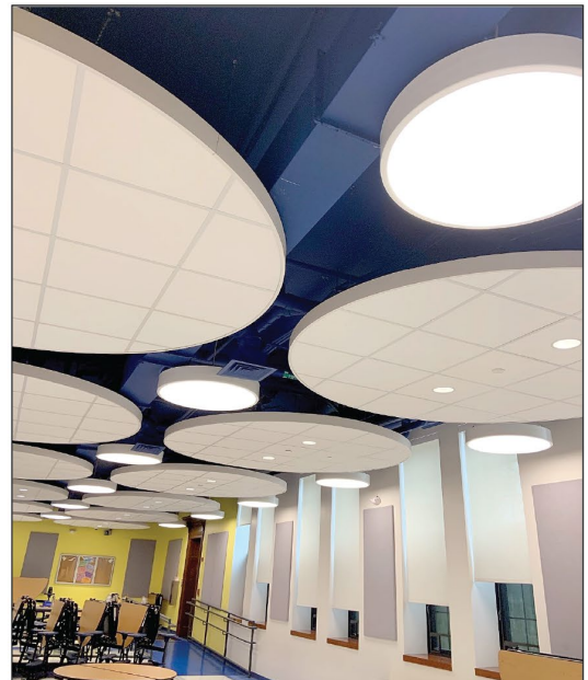
Acoustic shields on the ceiling to control cafeteria noise.
