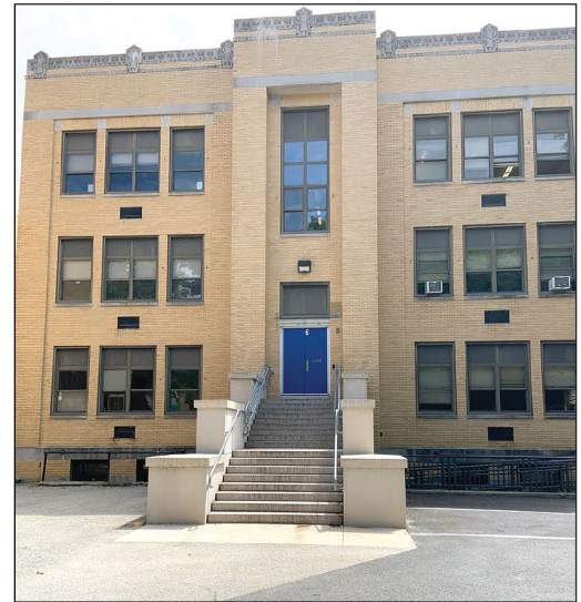
Main entrance is not accessible and school lacked signs directing people to an accessible entrance.
