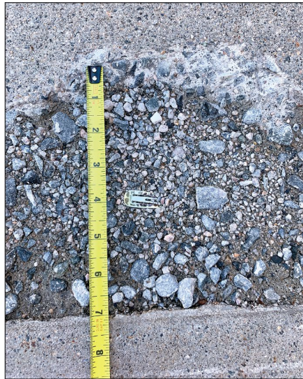
Uneven sidewalk surface with large holes found on path to school's main entrance.
