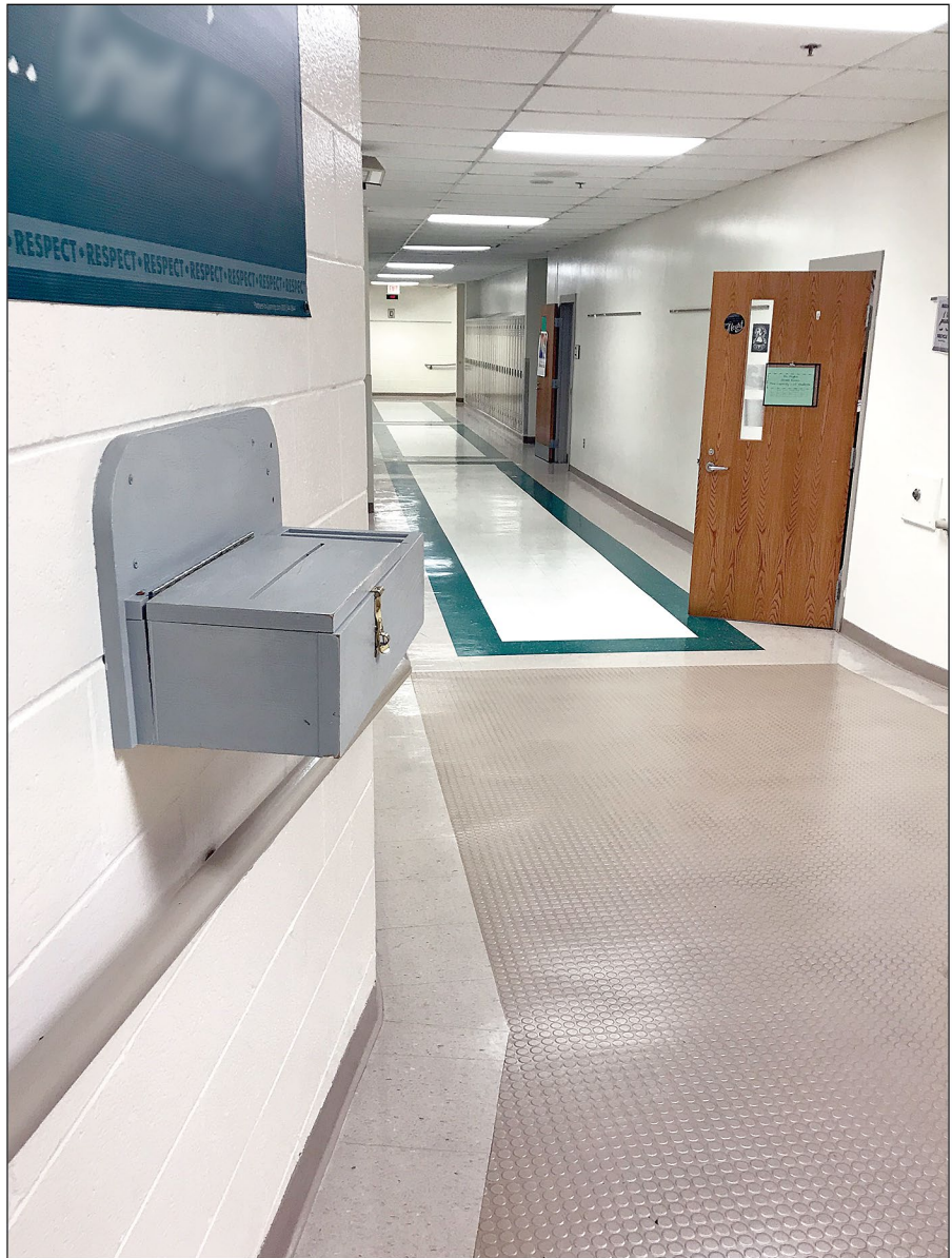
Protruding object in circulation path.
