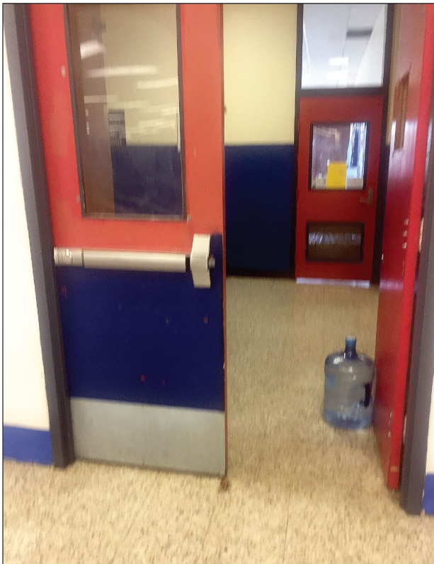
Propped-open doorway narrowed by a water bottle.
