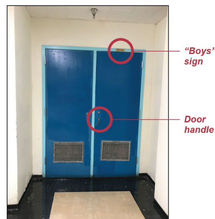
Restroom sign located too high, located on the door, and lacks raised characters or braille. Door hardware also requires pinching or grasping to open.
