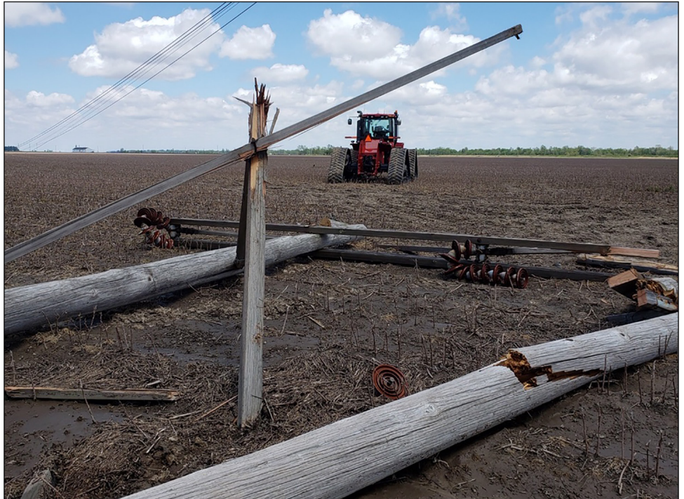
Figure 7: Strong Winds Damaged a Southwestern Power Administration Transmission Line (2020)
