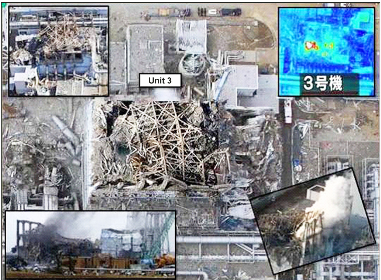
Figure 1: Unit 3 of the Fukushima Daiichi Nuclear Power Plant Following the March 11, 2011, Earthquake and Tsunami
