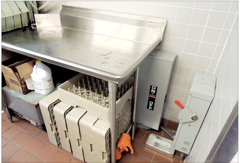
Figure 6: High Voltage Electrical Panel Installed Next to Cafeteria Dishwasher at a BIE-Operated School, October 2014
