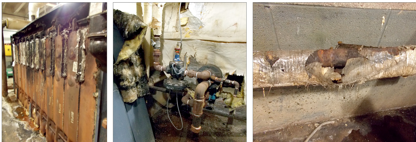
Figure 2: Aging Boiler Systems at a BIE-Operated School Built in 1959
