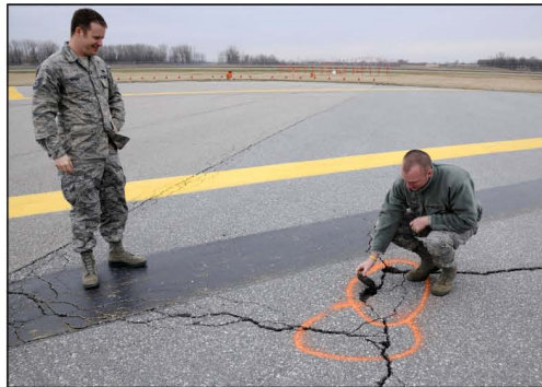
A servicemember marks a damaged area on an airfield flight line at Selfridge Air National Guard Base, Michigan.
