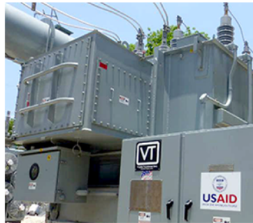
Port-au-Prince area electrical substation, April 2013
