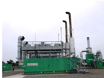
Caracol Industrial Park Power Plant, June 2014
