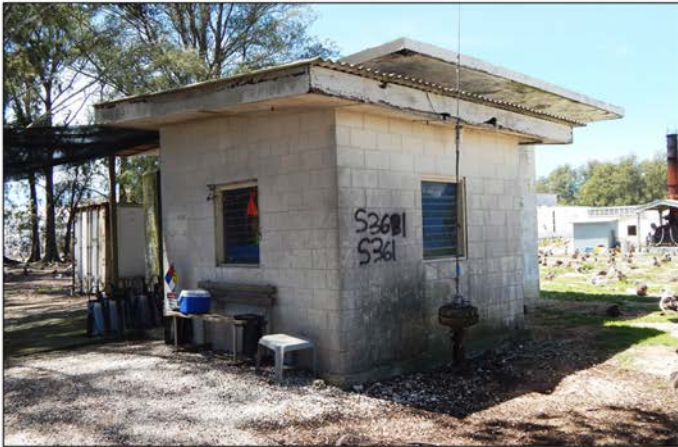
Figure 57: Electrical Switch Station (Property No. 361), Midway Atoll, Sand Island (April 13, 2015)
