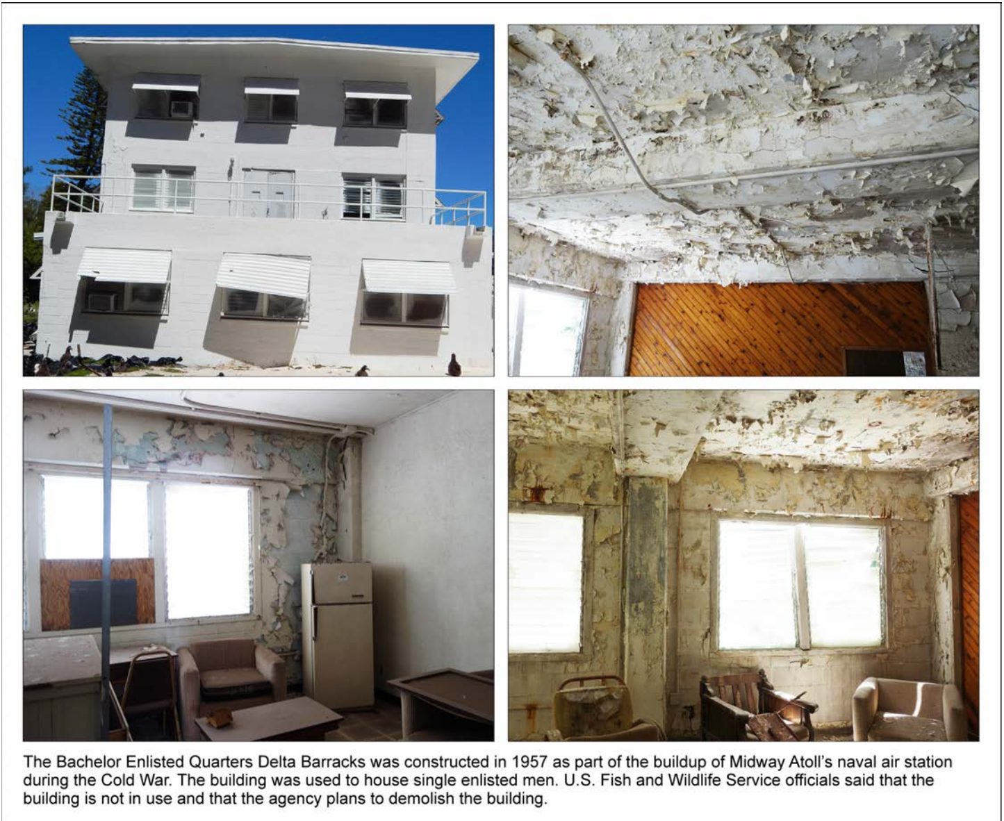
Figure 64: Bachelor Enlisted Quarters Delta Barracks (Property No. 3504), Midway Atoll, Sand Island (April 13, 2015, and April 17, 2015)
