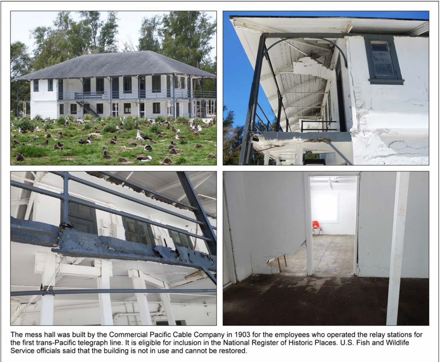
Figure 13: Cable Station Building, Mess Hall (Property No. 643), Midway Atoll, Sand Island (April 10, 2015, and April 17, 2015)
