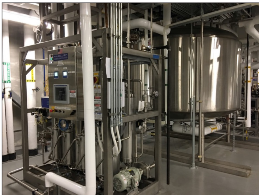
Water for injection generation system
