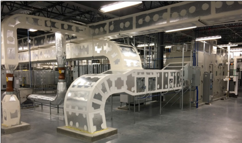
Air handler unit
