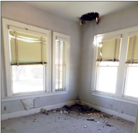
Interior damage of Kerrville Medical Center.
