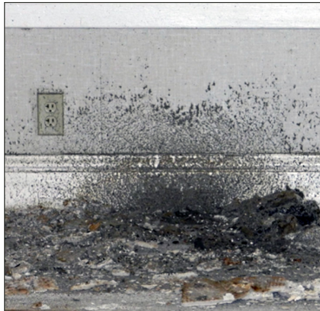
Portions of the ceiling have collapsed, spraying debris on to the floors and walls.
