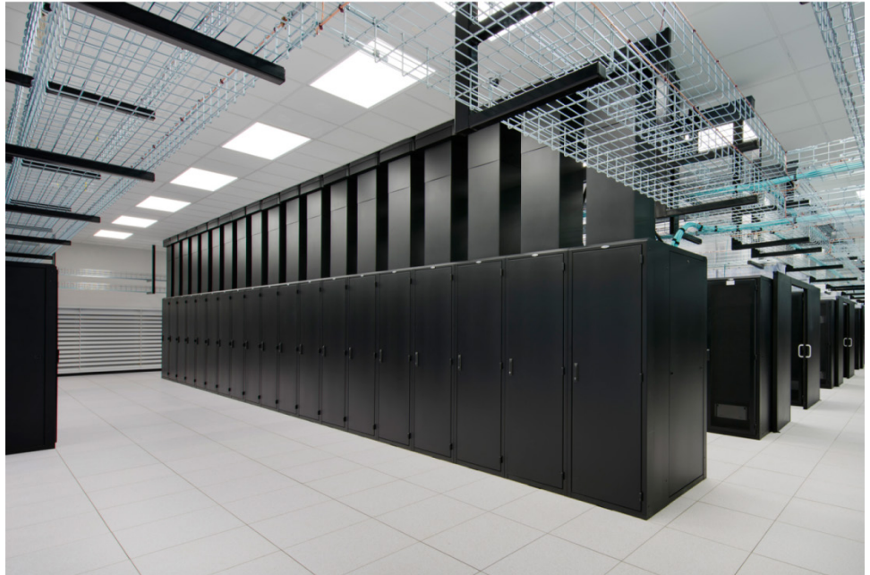
Figure 1: Example of Data Center Server Racks at the Social Security Administration's National Support Center
