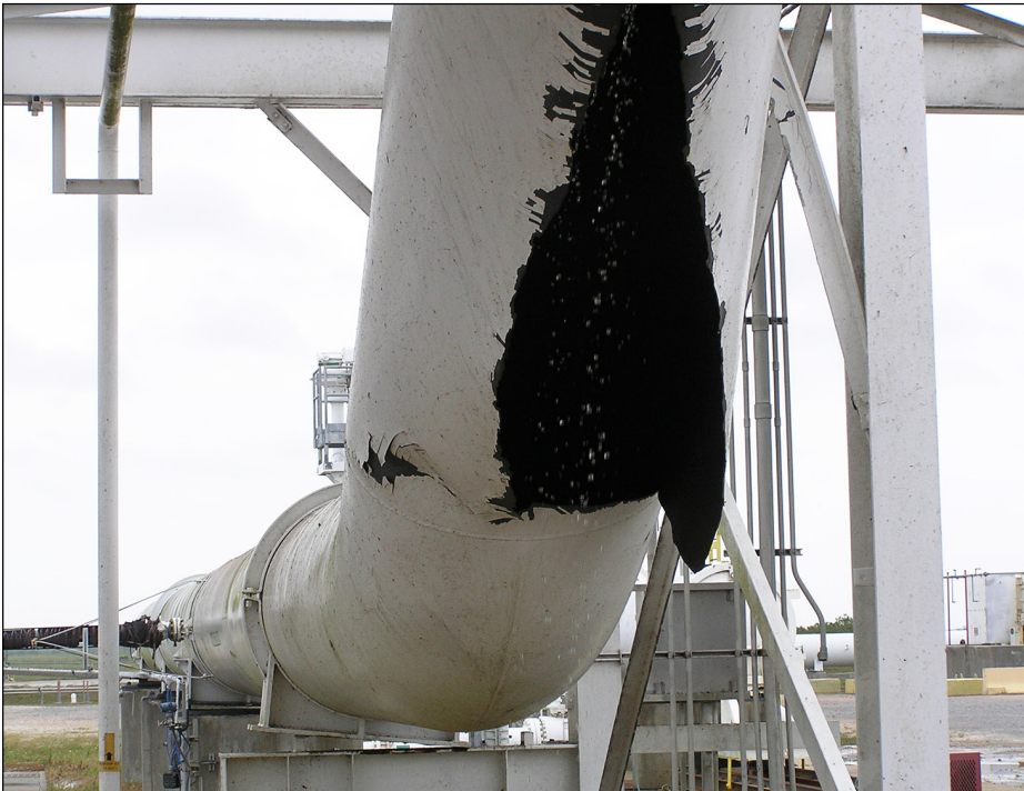
Figure 1: Strategic Petroleum Reserve, Big Hill Site – Raw Water Pipe Failure in April 2016
