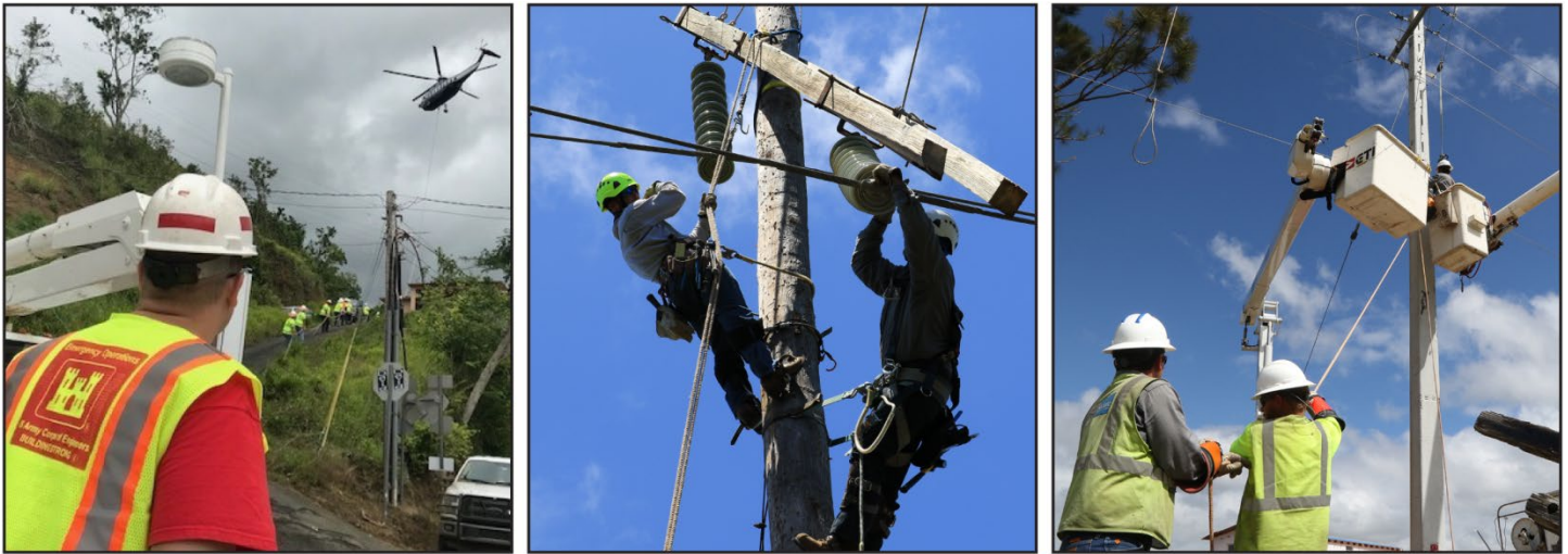
Figure 2: U.S. Army Corps of Engineers (USACE) and USACE Contractors Working to Restore Electricity in Puerto Rico
