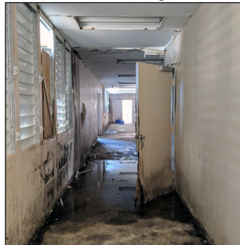
Interior damages to a school in Puerto Rico from water infiltration.
