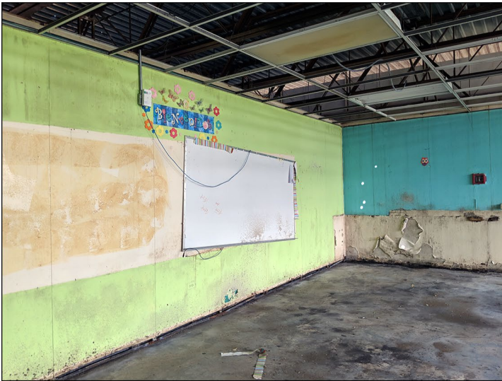
Classroom with molded floors and water damage on the walls at a school in San Juan, Puerto Rico.
