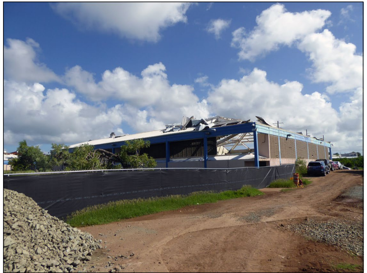
This school building in St. Croix sustained severe hurricane damage, including a collapsed roof.
