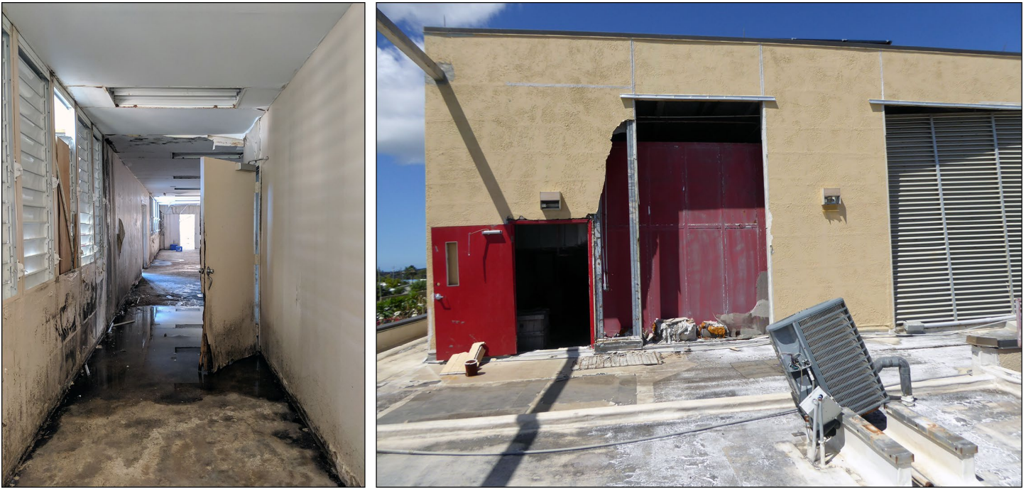
Interior damages to a school in Puerto Rico from water infiltration with standing water and molded walls. Damaged structure and ventilation system at a hospital in St. Croix.
