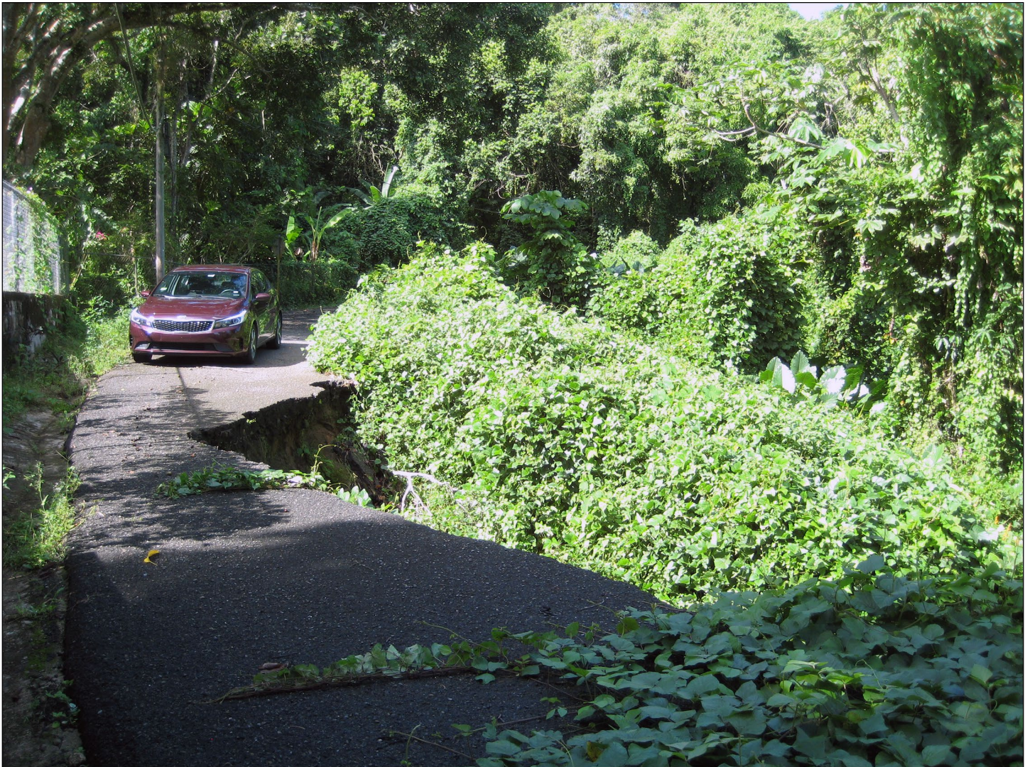
Figure 7: Collapsed Segment of Road Near Maricao, Puerto Rico, September 2018
