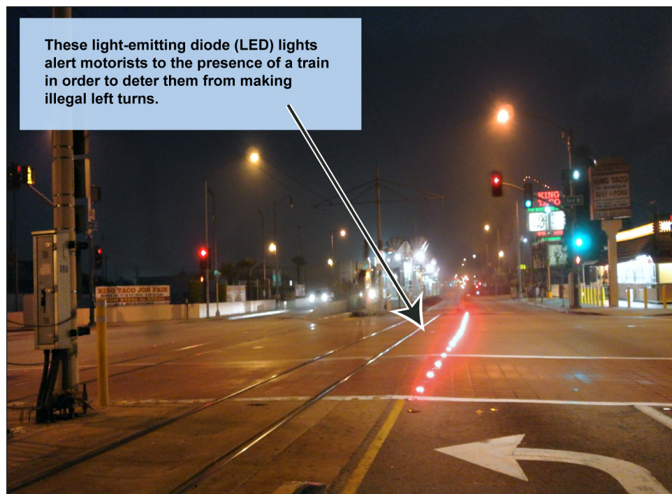
Figure 4: Photos of In-Roadway Lights That Delineate a Grade Crossing
