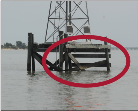
This damaged range/tower has been deemed unsafe to climb by an aids to navigation team.
