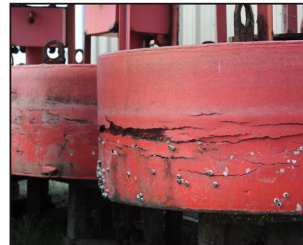
These 5' x 9' floating, foam buoys are showing deterioration from continued exposure to harsh maritime conditions.
