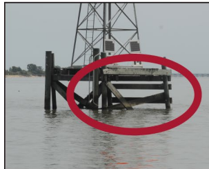
This damaged range/tower is in need of repair.
