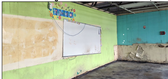
Classroom with mold on floors and water damage on the walls at a school in San Juan, Puerto Rico.
