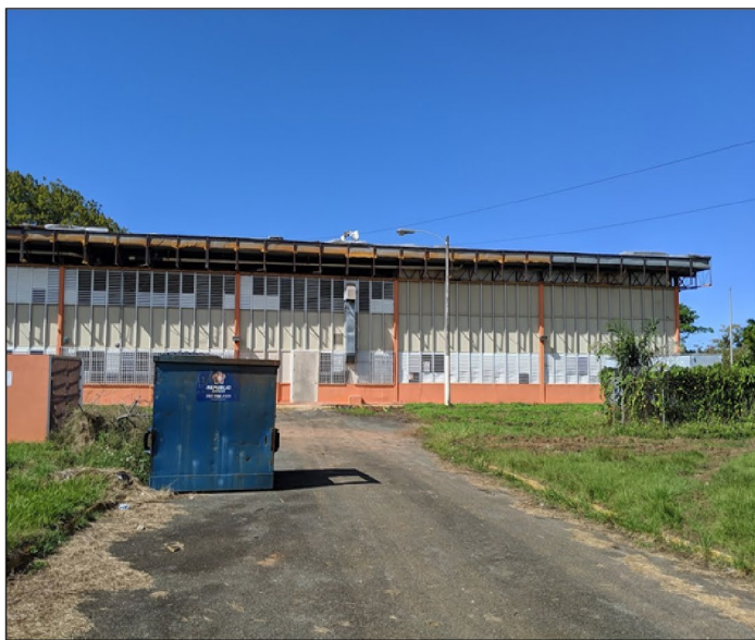
School with internal mold and water damages caused by Hurricane Maria observed in March 2019.
