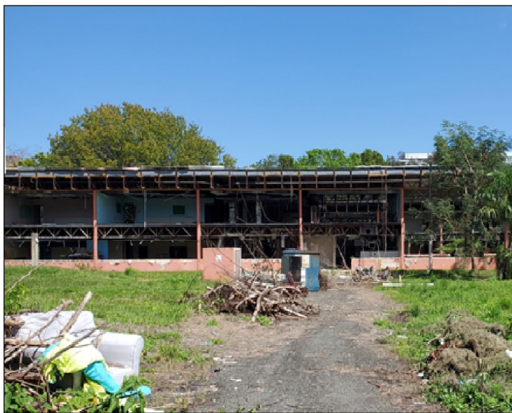
School observed in March 2022 awaiting repairs. According to a FEMA official, a construction crew removed doors, windows, and some walls due to asbestos and lead in the building.
