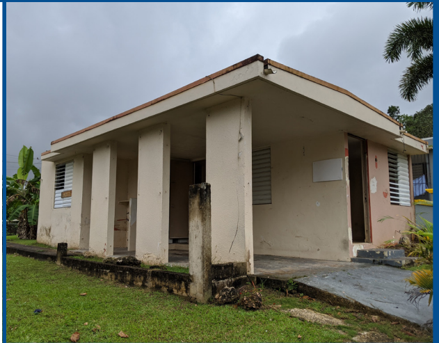
Damaged public housing unit in Puerto Rico, February 2020.
