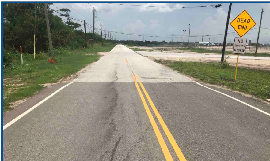
A Texas emergency highway repair project following Hurricane Harvey; repaired road built to updated design standards.
