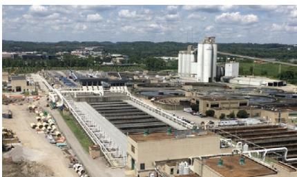
Central Wastewater Treatment Plant Capacity Improvements Project Source: Metro Water Services. | GAO-23-105285
