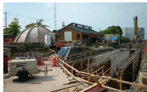
Excess Flow Management Facility Upgrade Source: City of Oswego, New York. | GAO-23-105285
