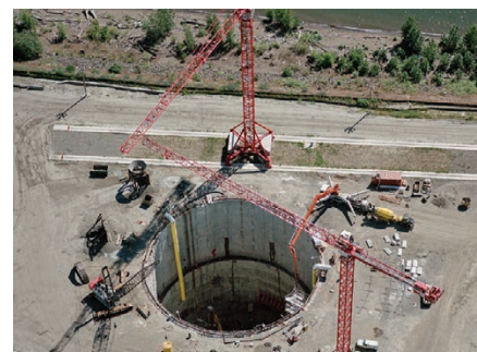
Work at the Swan Island CSO Pump Station as part of Portland's Big Pipe Project next to the Willamette River in 2004.
