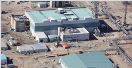
Source: GAO analysis of DOE documents and interviews with DOE officials; DOE (photo). | GAO-24-106014
