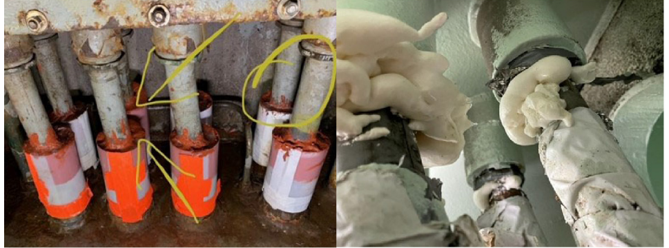
Figure 11: Use of Unauthorized Interventions, Including as Seen on Television Sealant Product and Plastic Wrap (left), Expanding Foam, Tape, and Common Store Bought Super Glue (right) as Documented by the Navy
