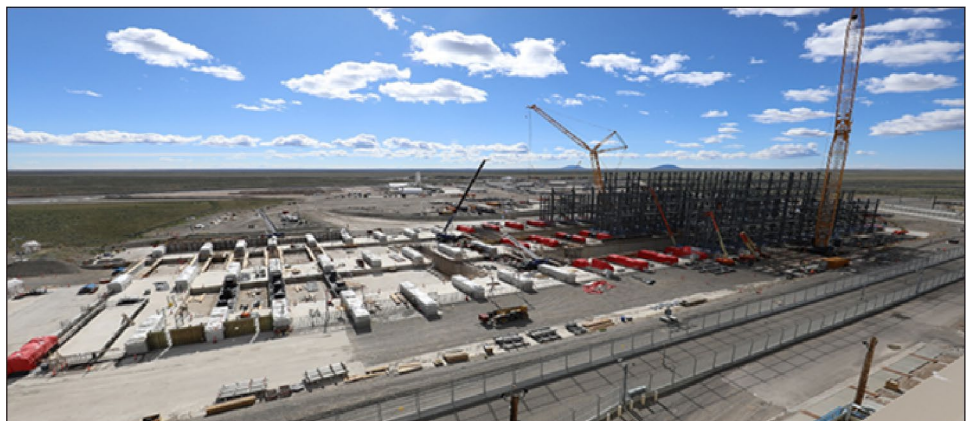
Figure 4: View of the Spent Fuel Handling Recapitalization Project (SFHP) Construction as of May 2024
