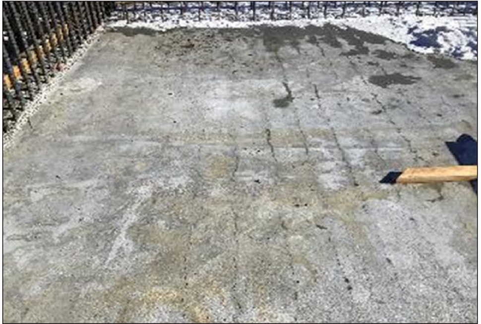
Figure 6: Spent Fuel Handling Recapitalization Project (SFHP) Concrete Foundation Cracking
