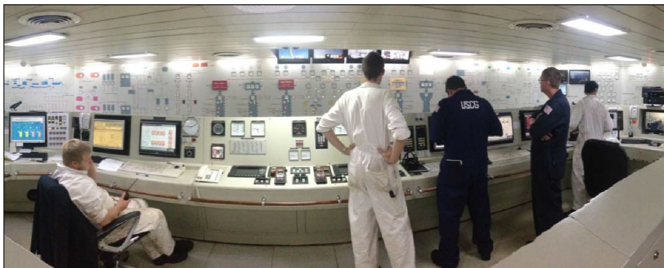
Figure 3: Engine Control Room of a Modern Cruise Ship
